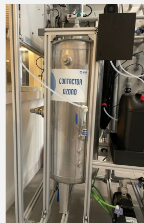
Ozone contact reactor Ozone destruction system: Thermocatalytic
